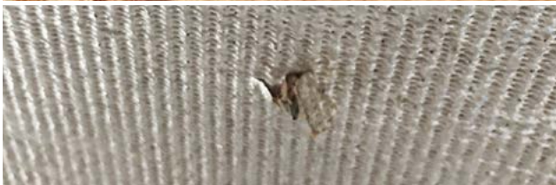
Roofing nails piercing roof decking
